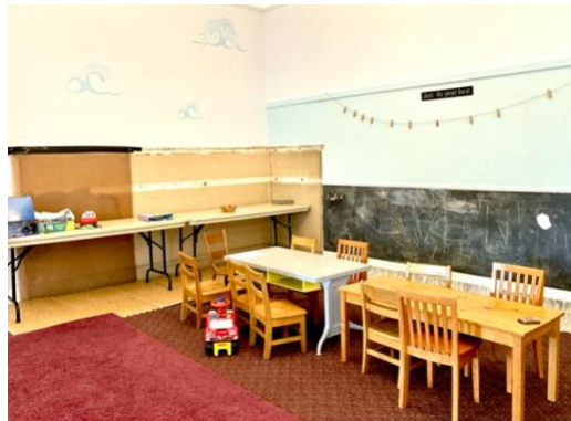
Photo: As of 7/22, cabinets have been removed from the southwest corner to make room for a hand-washing sink.
